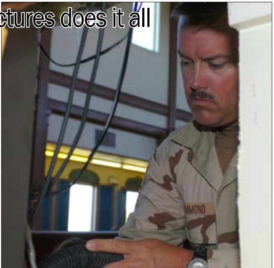
Air Force Master Sgt. Stephen Hammond, shop manager, vacuums drywall and sawdust out of the sound booth in the NAVSTA chapel during a project to create an access door to the wiring system behind the soundboard. – JTF Guantanamo photo by Army Staff Sgt. Emily J. Russell
