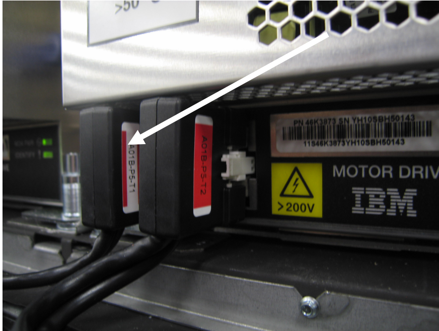
Figure 14 WCU MDA Power Cable labels
