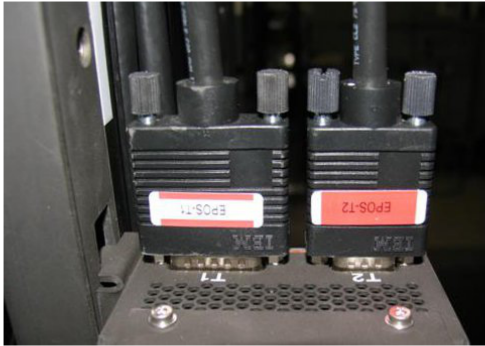
Figure 4 UEPO Panel Cables Plugged
