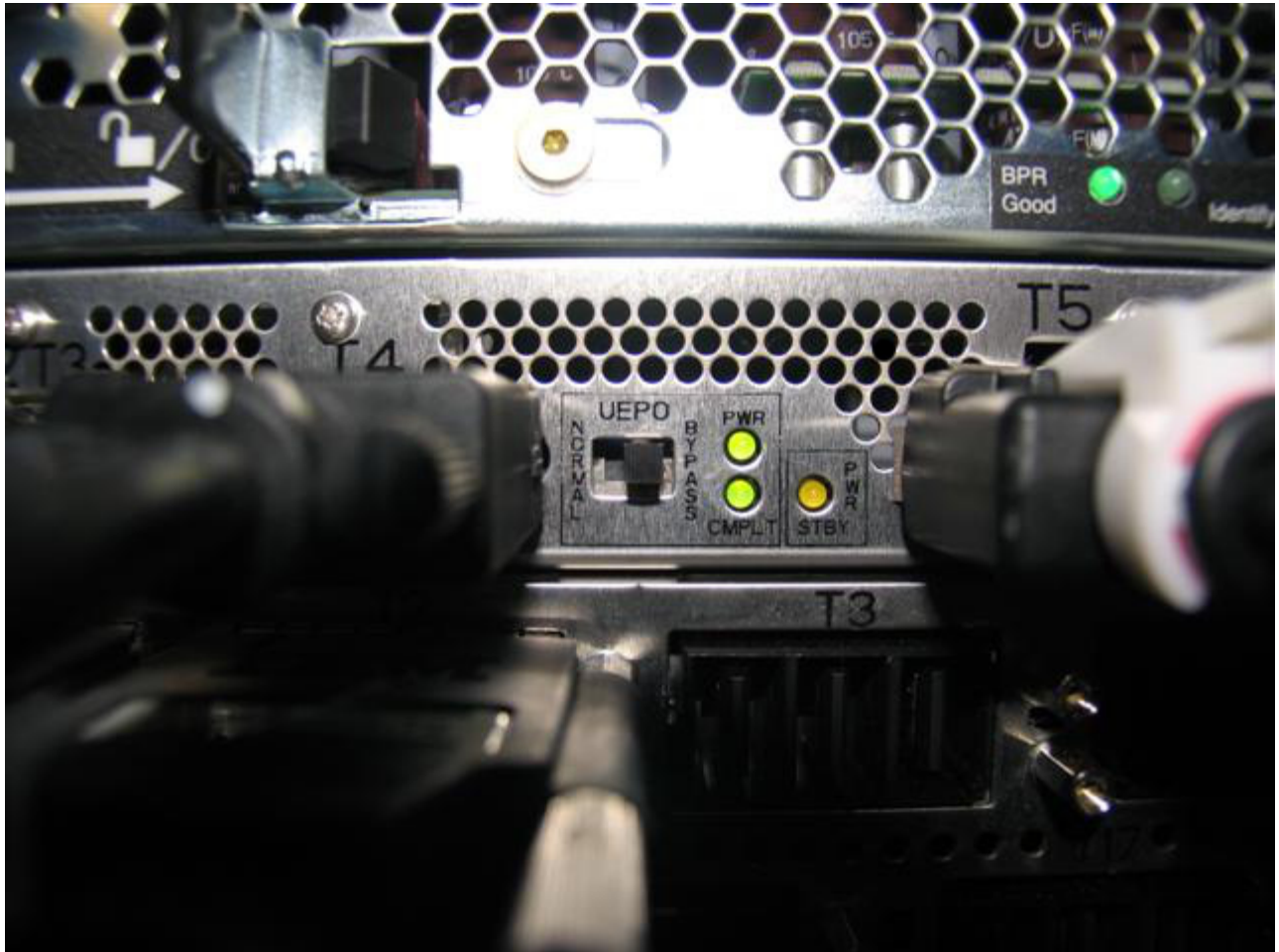
Figure 12 BPC UEPO Bypass Switch shown in desired BYPASS position (moved to the right)
