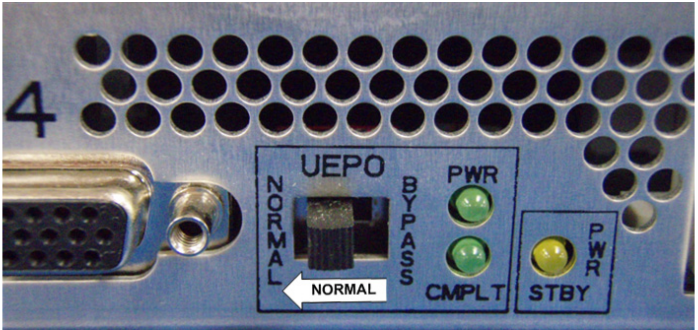
Figure 16 BPCH UEPO Bypass Switch shown in the desired NORMAL position (moved to the left)
