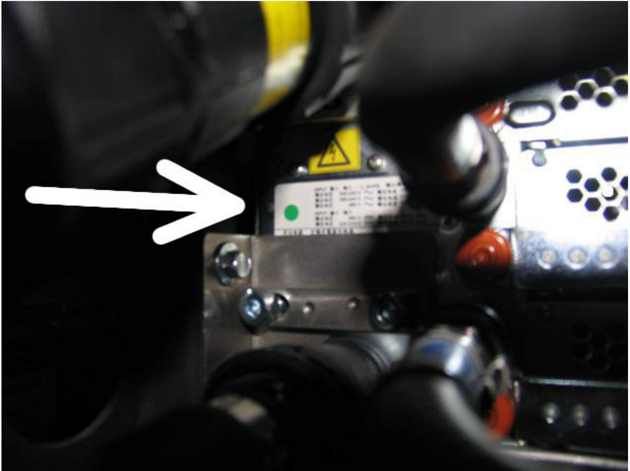
Figure 19 Power Cord/Flexible Power Cable LED shown not lit due to wall CB turned off
