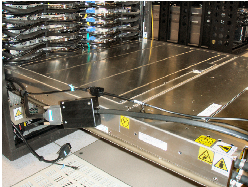
Figure 26 Left HPIC and Ethernet Test cables connected to Rack Cables
