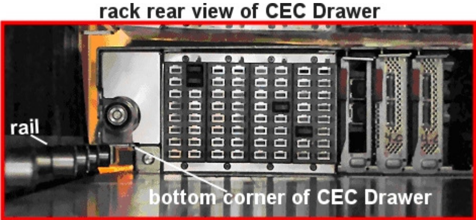
Figure 2 CEC Slides/Rails in rack
