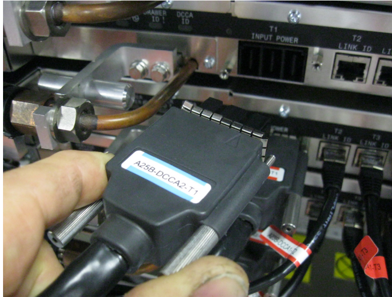
Figure 14 Typical HPIC Cable
