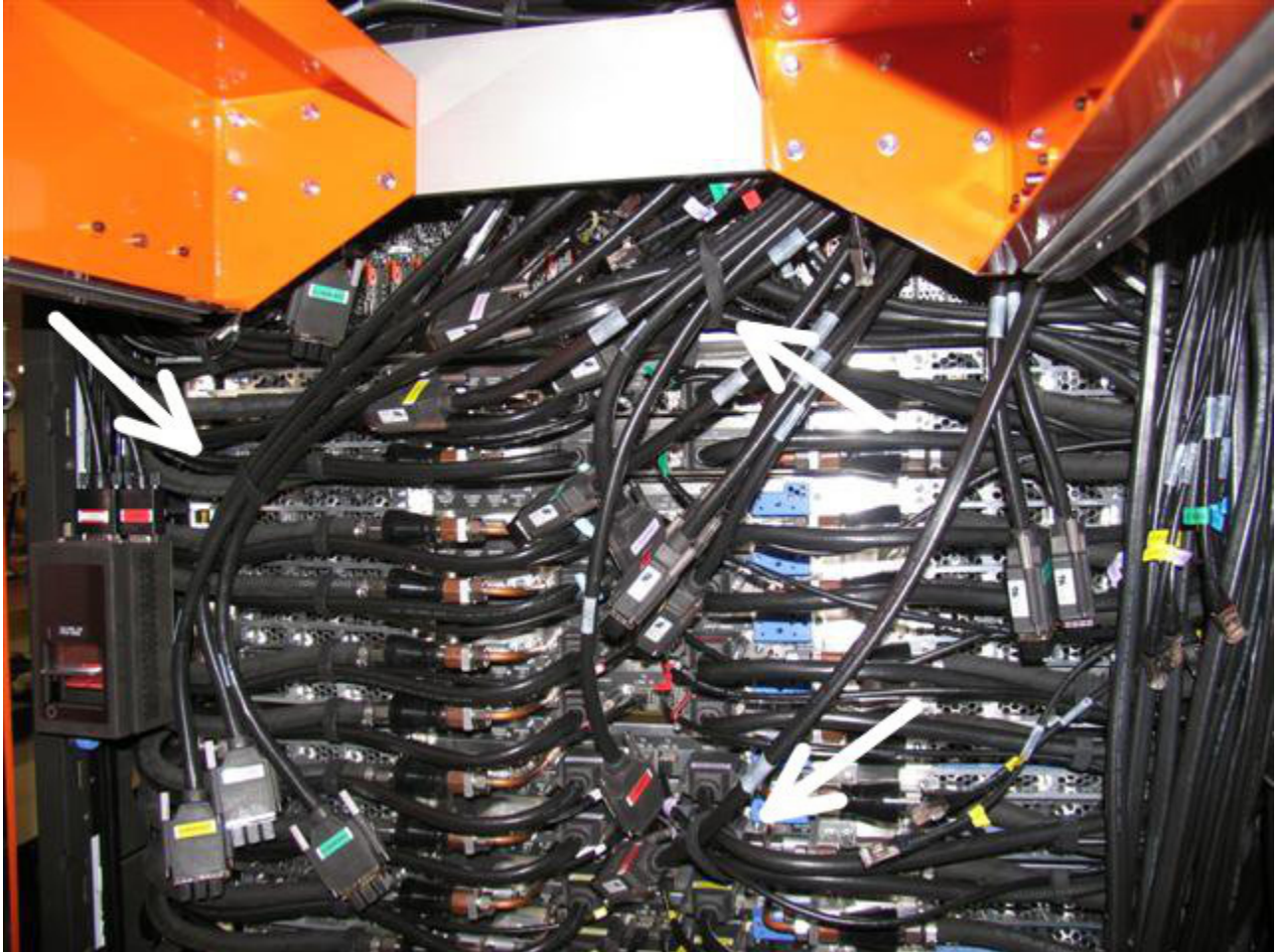
Figure 23 BPE-B Cables Dressed/Secured Clear of Lift Tool (Larger configuration)
