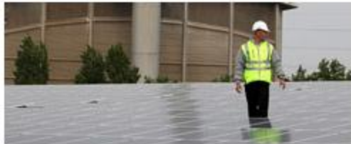
Solar panels fitted at our Beckton site
