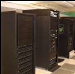
smarter data center
