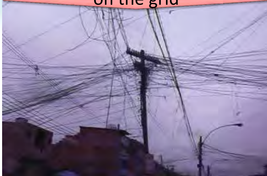
Irregular connections on the grid
