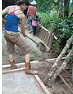
Fig. 9f: Carrie Schaden burying the tank bound pipe to allow a footpath
