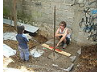
Fig. 7: Zach and Juanito checking the level of the tamped area for tank
