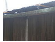
Fig. 12e: Gutters fail test
