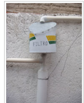
Final debris filter
