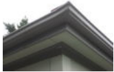
Fig 1: This is the original gutter siding that later had a downspout put into it for the water to come out
