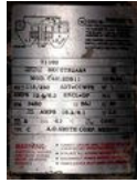
Figure 3: Pump label. No additional flow rate information could be found from the information on this label.
