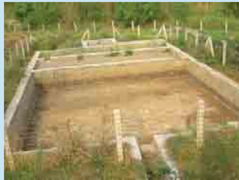
Leachate collection tank
