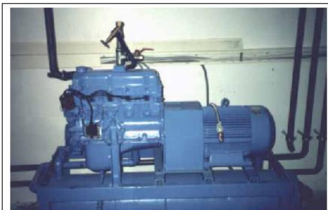
Figure 47: Co-generation unit (electricity and heat utilisation)
