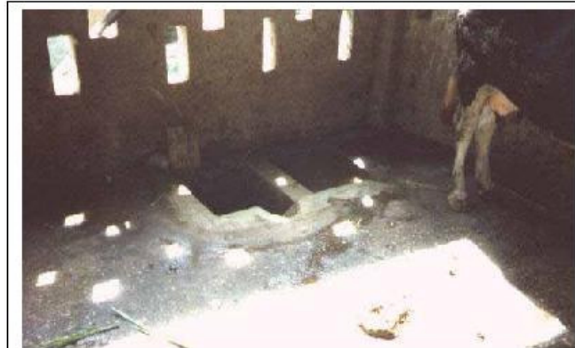
Figure 23: Cowshed, directly connected to the plant: A urine chamber to the right collects the liquid which can be used to wash the dung into the digester.
