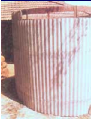
Fix the galvanised iron (GI) sheets to the mould and cover them with
