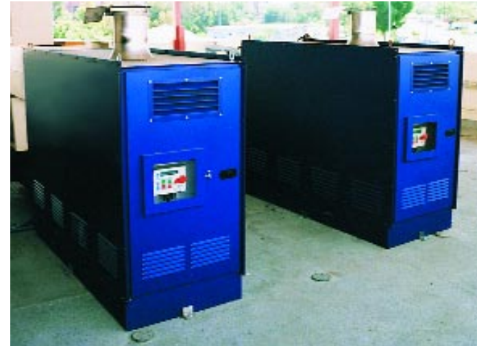
Two micro-turbines under endurance testing at ETS' test facility
