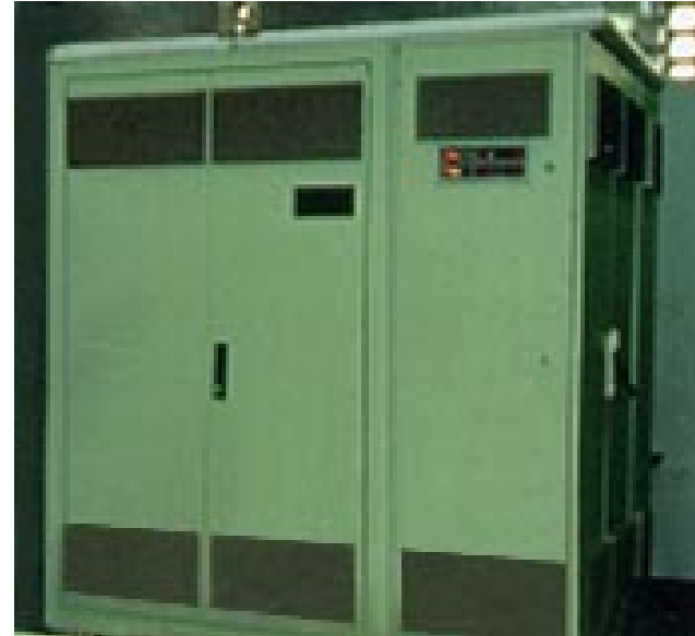
Prototype 25 kW SOFC in operation at the National Fuel Cell Research Center at Irvine, California. ETS is a founding member.
