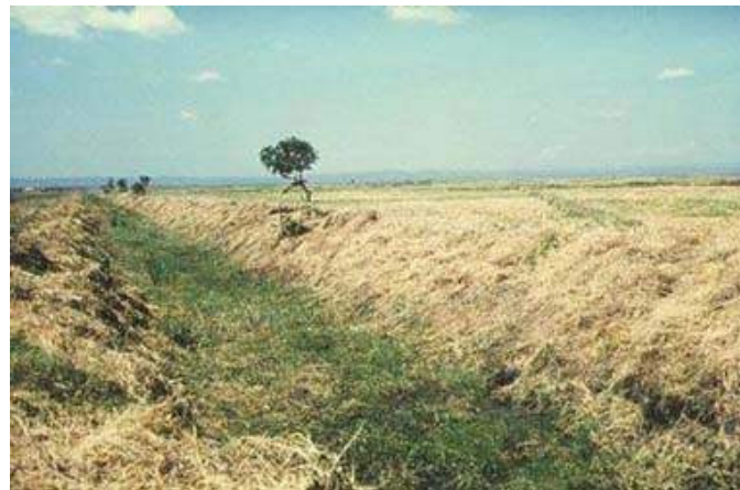
Slide J.22 Drying out of canals
