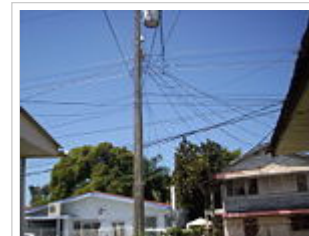
In Honduras electricity comes in to households through overhead cables. Other cables carry telephone, cable television and broadband internet.
