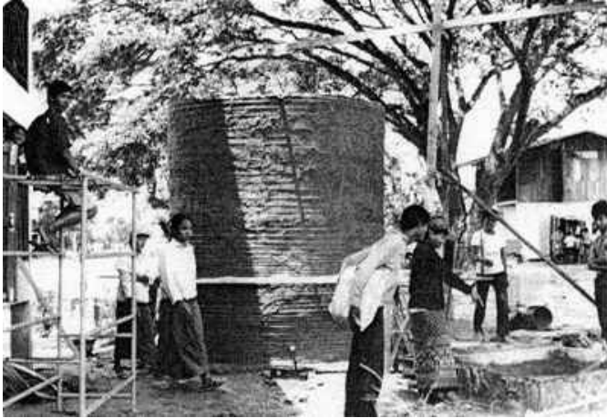
Figure 2 - a partially finished brick tank showing external rendering and hoop reinforcement (Chayatit Vadhanavikkit)
