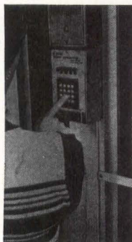
Fig 2 Building personnel must enter unique identification numbers into keyboard before entering. Microcomputer checks memory to determine if person is authorized to enter building at that time of day (or day of week) and unlocks door if person is entitled to enter
