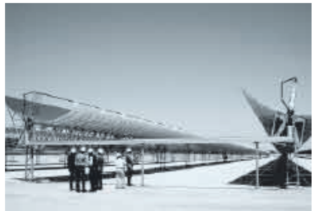
SKAL ET Parabolic Trough Collector loop, built by Solar Millennium AG and FlagSol into the operating SEGS V plant at Kramer Jct., California.
