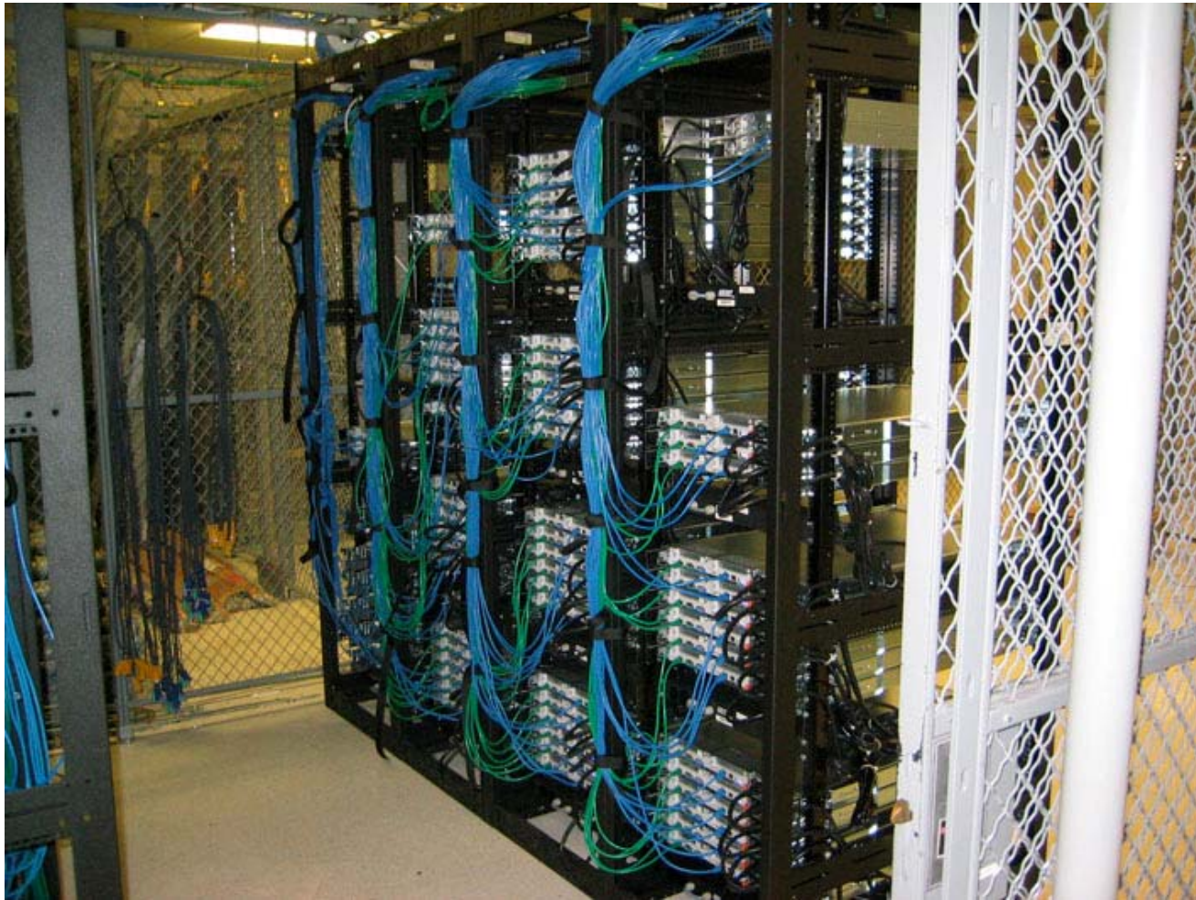
One of our cages in Tampa facility (350 Linux servers, in Florida, Amsterdam and Seoul)
