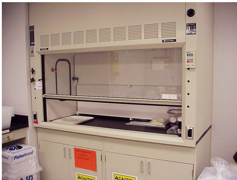
Figure 1.24: A laboratory fume hood. This laboratory hood sucks dangerous fumes out of a lab and allows researchers to work with dangerous chemicals without breathing them. (27)
