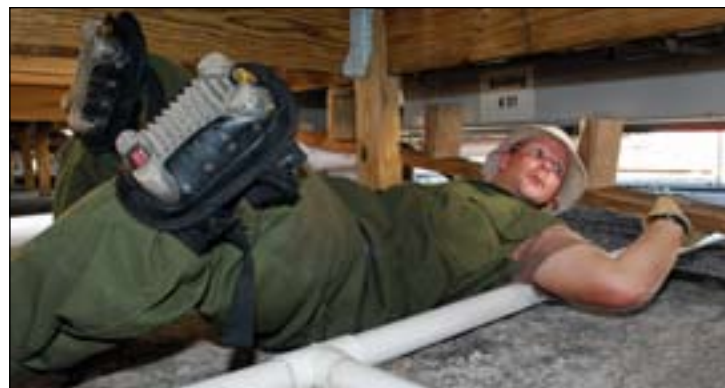
Air Force Staff Sgt. Sean Swiatocha, a structures sergeant, 474 th ECES, lifts a wooden brace crafted here to support the housing deck above, Nov. 13.
