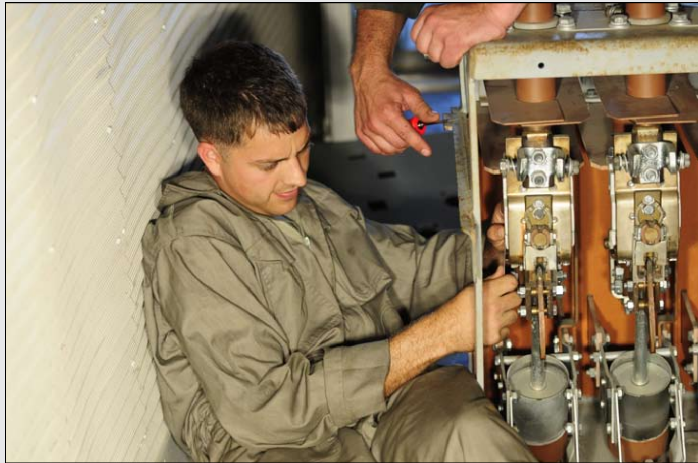
Steelworker 1st Class Shawn Heer of the Port Hueneme, Calif.-based Mobile Utilities Support Equipment Team works on a circuit breaker of a generator, Feb 3. — photo by Mass Communication Specialist 2nd Class Elisha Dawkins
