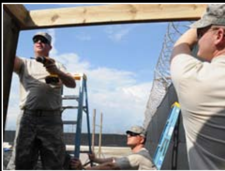
Staff Sgt. Jim Charles (left) examines a screw he fastened into a rafter while Senior Airman Matthew Frost supports the rafter as part of the construction of an awning adjoined to the guard shack at the entrance of the Expeditionary Legal Complex near Camp Justice, Tuesday. — photo by Mass Communication Specialist 2nd Class Jordan J. Miller
