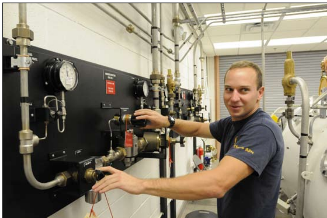
Navy Diver Third Class Nicholas Barna opens a series of valves to bring the decompression chamber online. The chamber is kept in a modified standby mode that allows the system to be completely operational in less than ten minutes.
