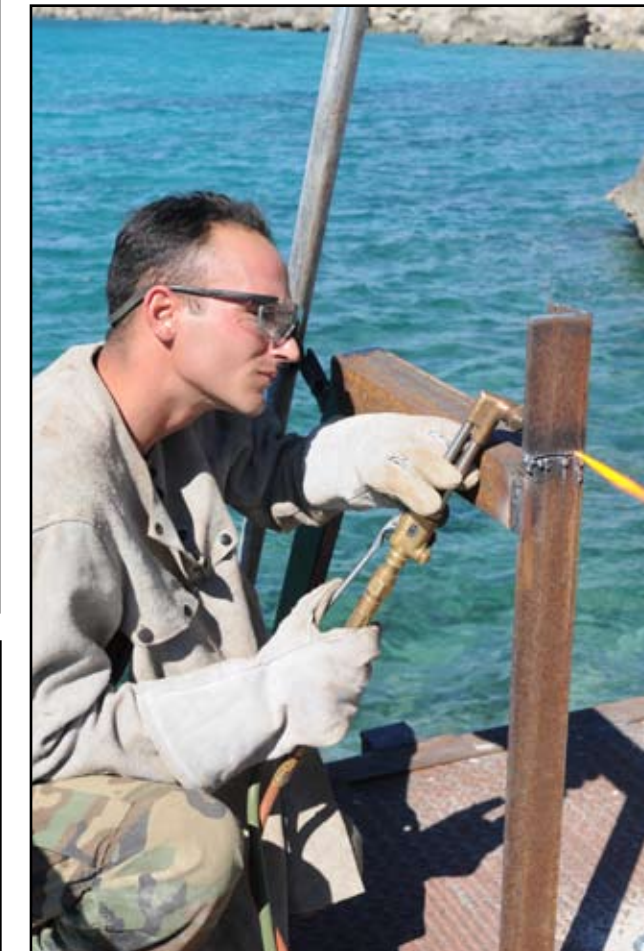
Navy Petty Officer 2nd Class John Blake welds steel beams to a railing at Phillips Dive Park.
