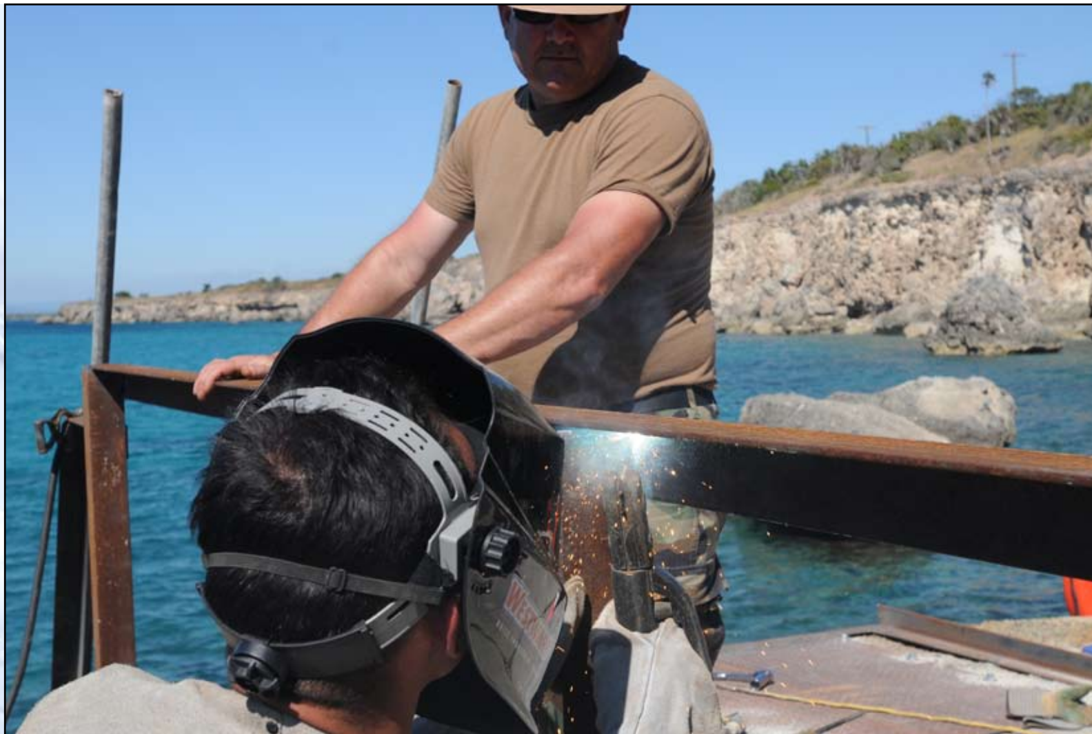
Petty Officer 1st Class Rex Miller observes Navy Petty Officer 2nd Class John Blake welding during reconstruction of a dive spot demolished during a recent hurricane.
