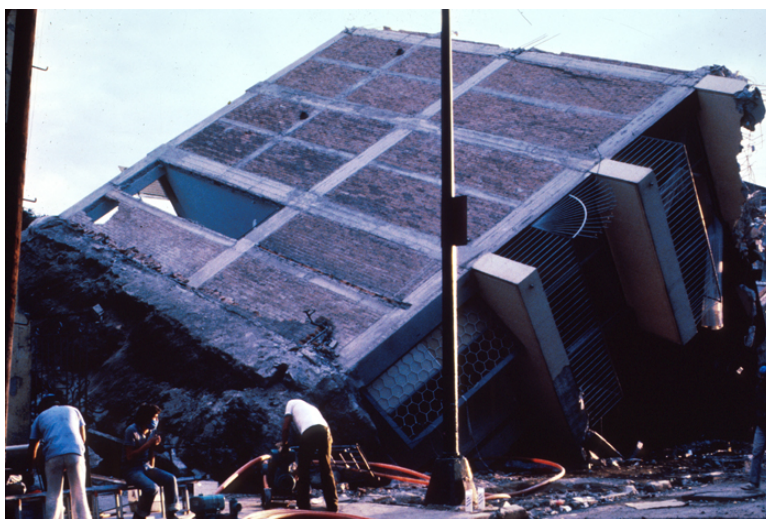
Figure 7.45: Liquefaction of sediments in Mexico City caused the collapse of many buildings in the 1985 earthquake. (9)
