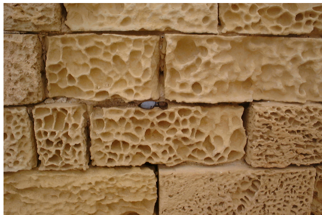
Salt weathering of building stone on the island of Gozo, Malta.
