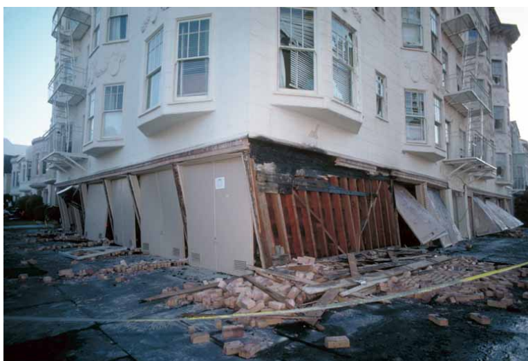
Figure 7.47: The first floor of this San Francisco building is collapsing after the 1989 Loma Prieta earthquake. The building is being held up by the two walls that are not in the photograph and the strength of the upper floors. The two walls that are in view are not strong because they had doors in them. (42)
