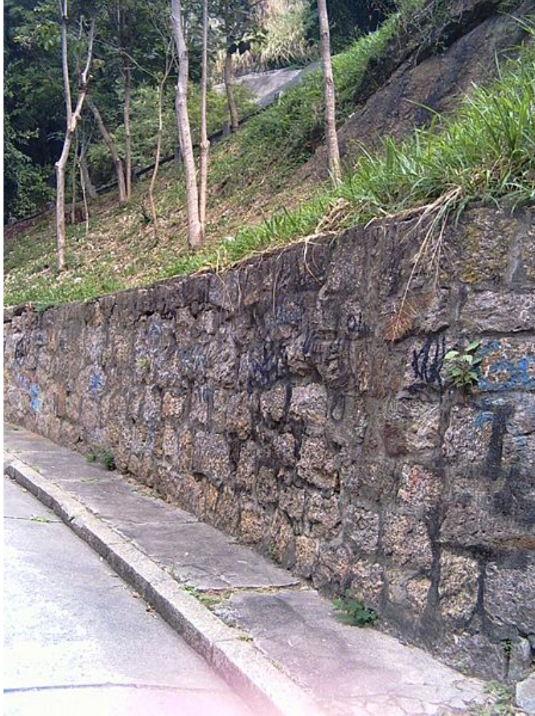
Figure 10.47: It is important to reinforce a slope that has been cut away in order to prevent landslides. (19)
