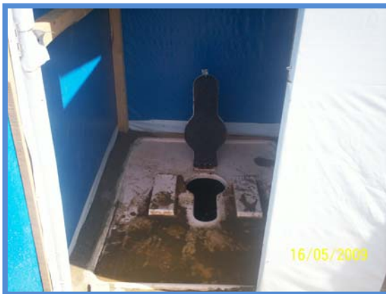
Figure 16. Dry toilets are now started giving problems
