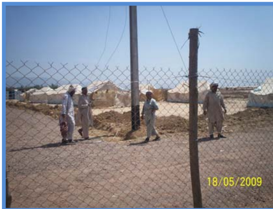
Figure 25. Electrification at Jalozai camp
