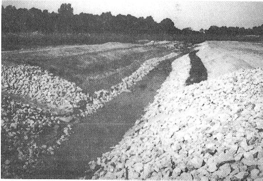
Figure 7-11. Riprap placed along a drainage channel for protection against erosion.
