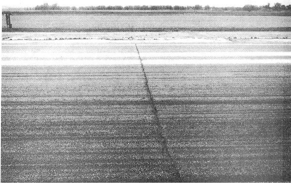
Figure 3-8. Transverse reflective crack.
