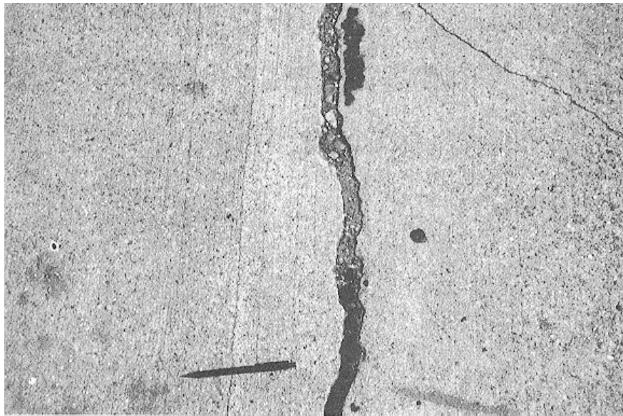
Figure 4-10. Joint seal damage, incompressibles in joint.
