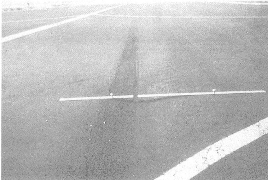
Figure 3-4. Sag in asphalt pavement.
