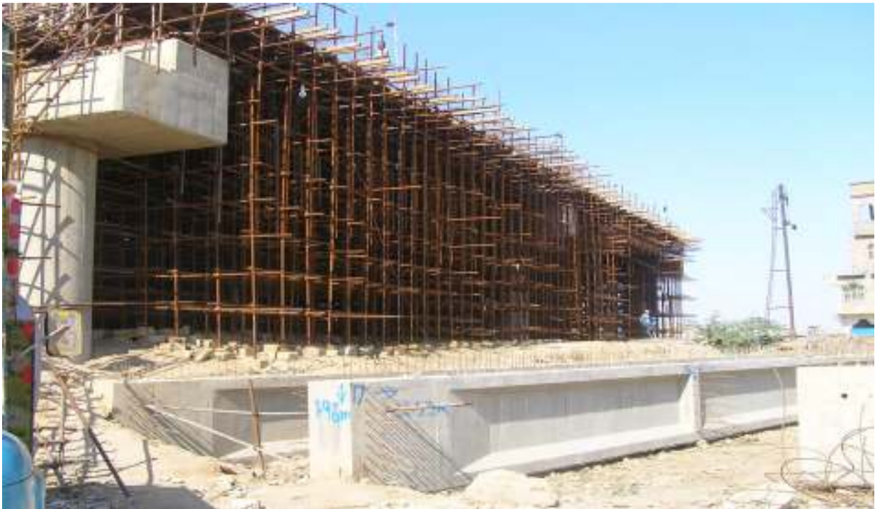
Leyari Expressway, Sir Shah Suleman Interchange, Grid 1 to 2, South Bound Box Girder, Form Work (Karachi-Pakistan) Side View Sultan Mahmood and Company Engineers and Contractors
