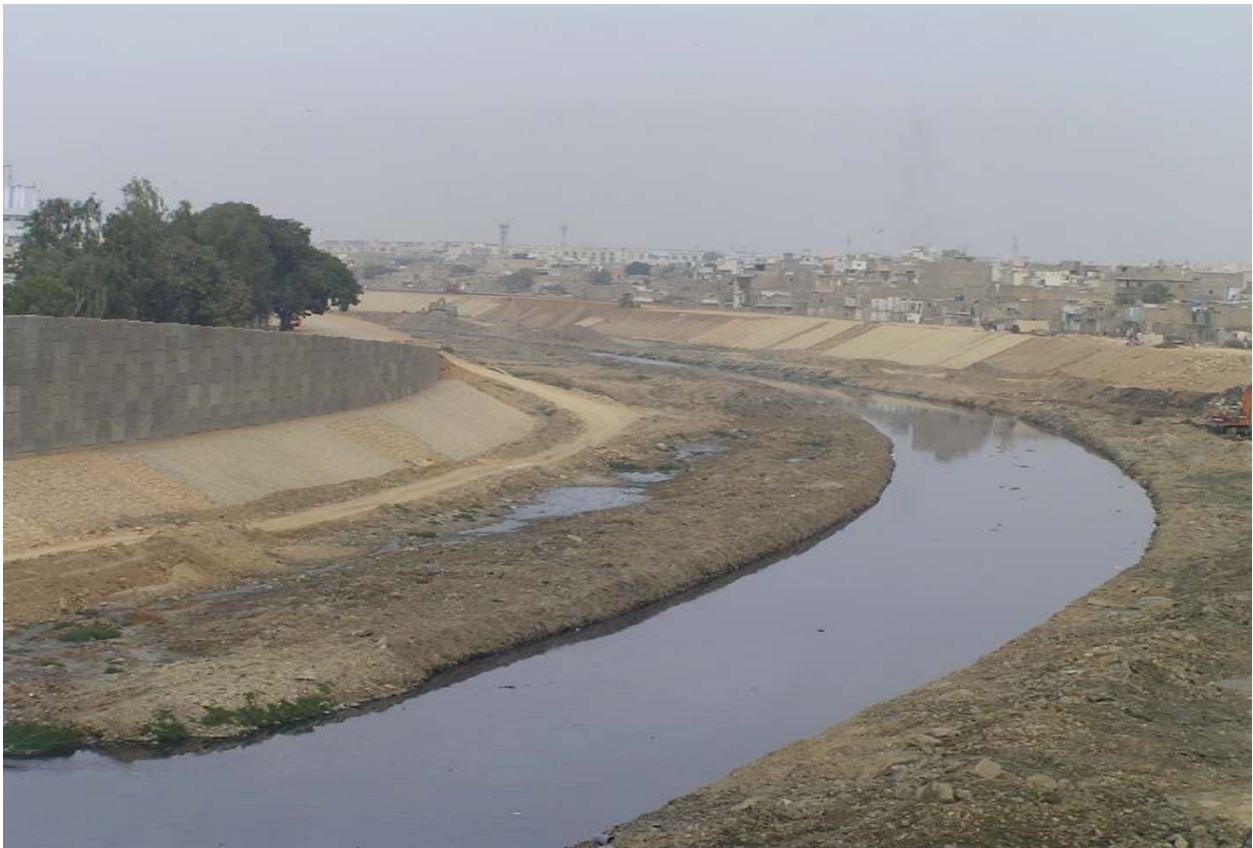
Leyari Expressway, Shorab Goth, Dredging Work (Karachi-Pakistan) Sultan Mahmood and Company Engineers and Contractors
