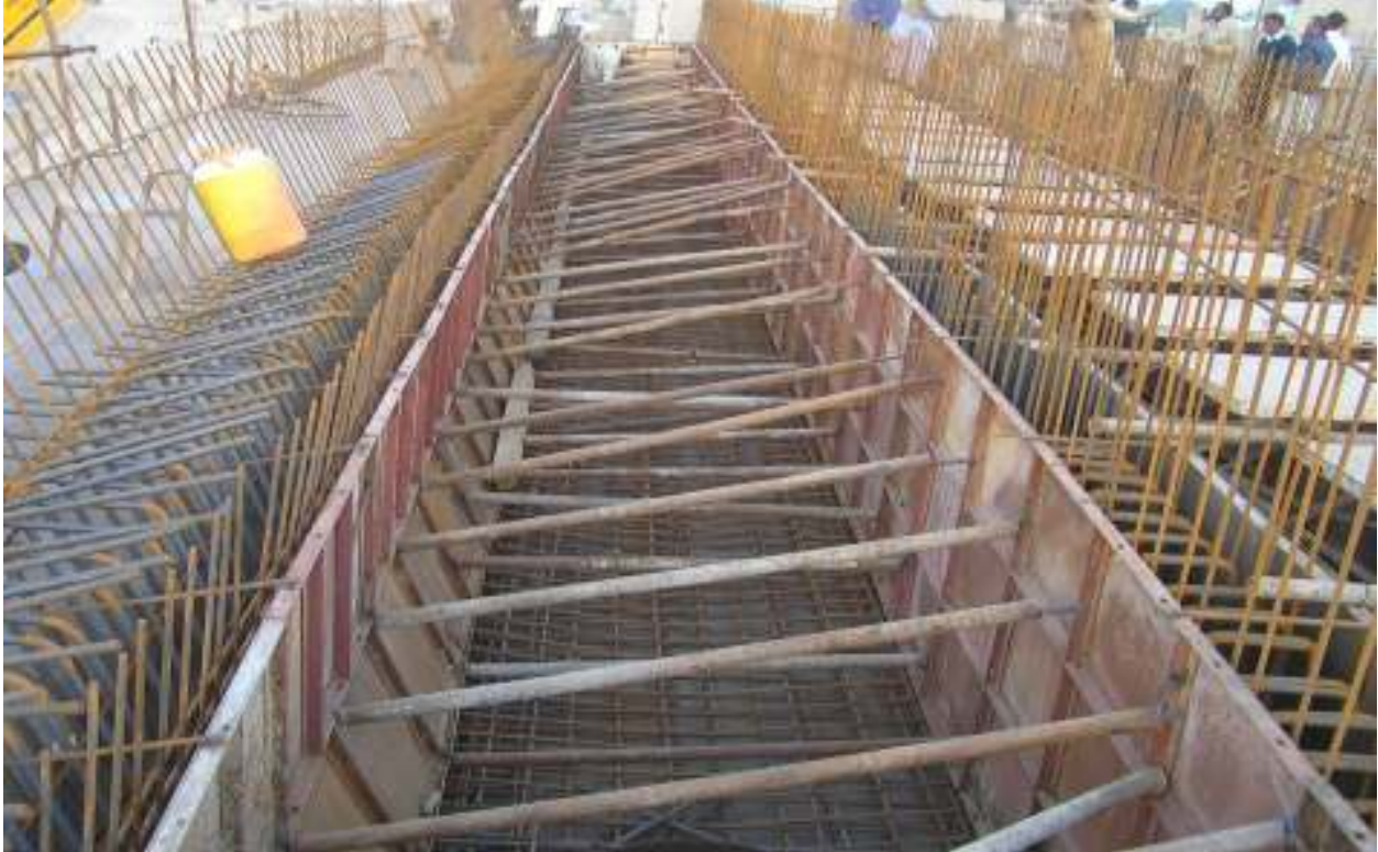
Leyari Expressway, Sir Shah Suleman Interchange, Grid 1 to 2, South Bound Box Girder, Form Work (Karachi-Pakistan)
