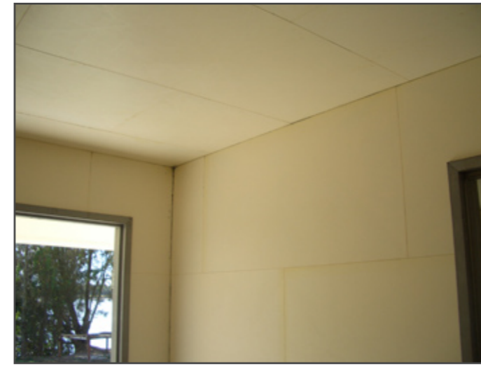
Unflushed Walls & Ceilings
