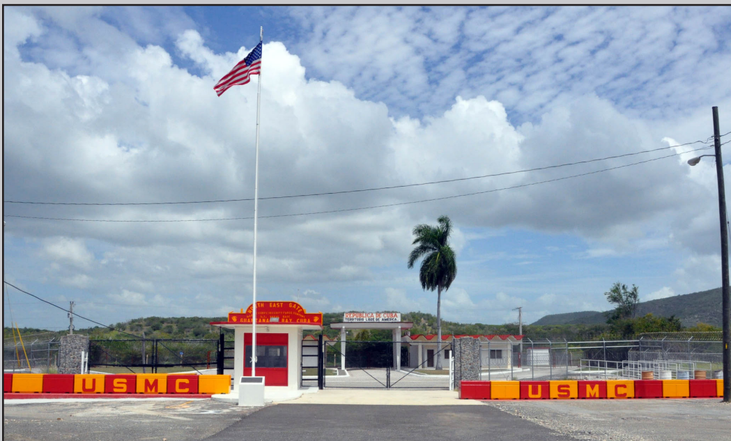
The North East gate after an approximately $70,000 renovation project including fresh paint, new concrete, and the removal of debris. The upgrade was facilitated by four Seabees attached to NAVFAC Southeast PWD and NMCB 23 and took more than 300 hours to complete.
