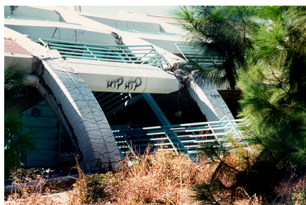
A collapsed parking structure at 1994 Northridge earthquake [1]
