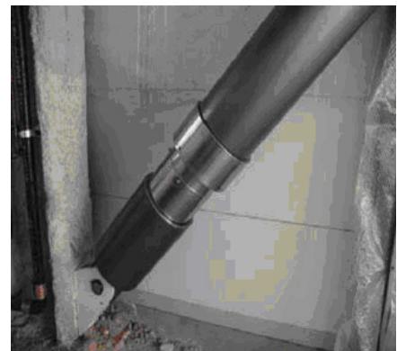
Fluid viscous damper installed in a building structure
