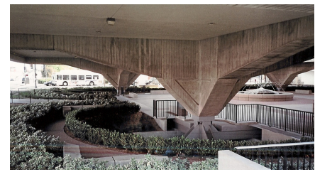
Bottom view of the Municipal Services Building [1] sitting on abutments of its elevated building foundation, Glendale, CA
