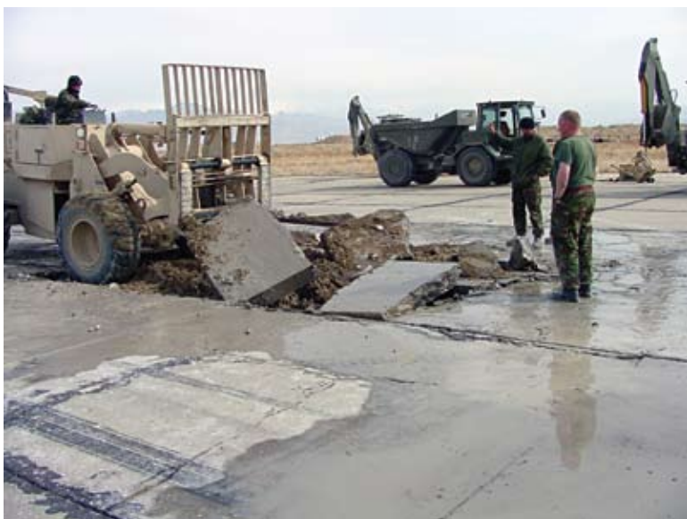
The removal of broken concrete slabs was the first step to repairing the damaged runway.
