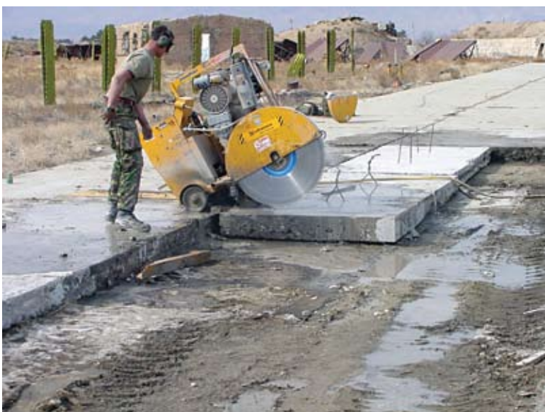
Special concrete saws were used by the engineers to cut the broken slabs into sections before removal.
