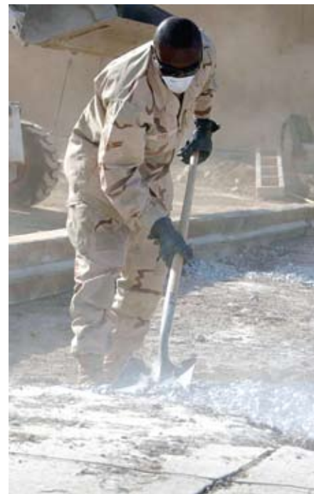
The U.S. Air Force’s Red Horse Squadron arrived in August 2002. The Red Horse Squadrons specialized in runway repair.
