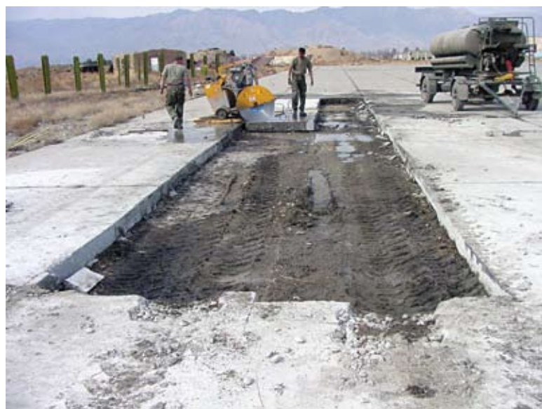
Extensive excavation was required before new runway slabs could be poured. The landing of heavy cargo aircraft necessitated a major runway repair effort at Bagram.
