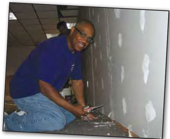
Mike Goodwin at work during the United Way Day of Caring. He and others were helping to construct a community center.
