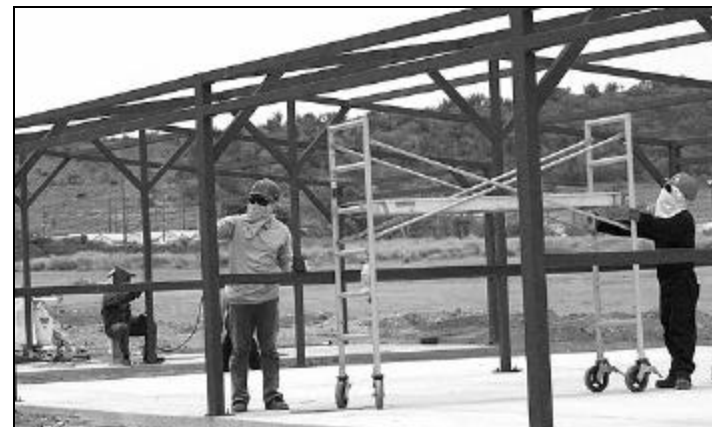
A work in progress: Brown & Root workers weld and paint joints on the frame of a Camp America North barracks-to-be. This structure is currently scheduled to be completed in October.
