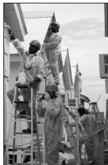
Brown & Root workers put a coat of sun-reflecting white paint on the SEAhuts at Camp America.
