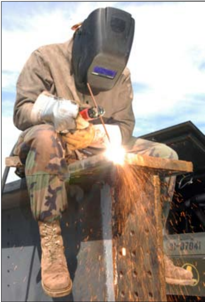
Navy Petty Officer 3 rd Class Matthew Long, a steel worker with Naval Mobile Construction Battalion Four, cuts through a metal support of a bridge under construction here, Nov. 7. – JTF Guantanamo photo by Army Spc. Erica Isaacson
