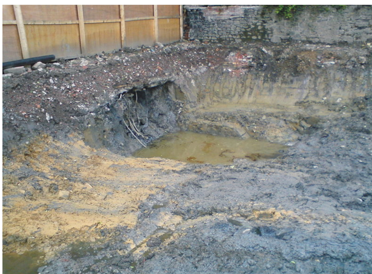
Figure 25.32: Soil contamination caused by underground storage tanks containing tar. (8)
