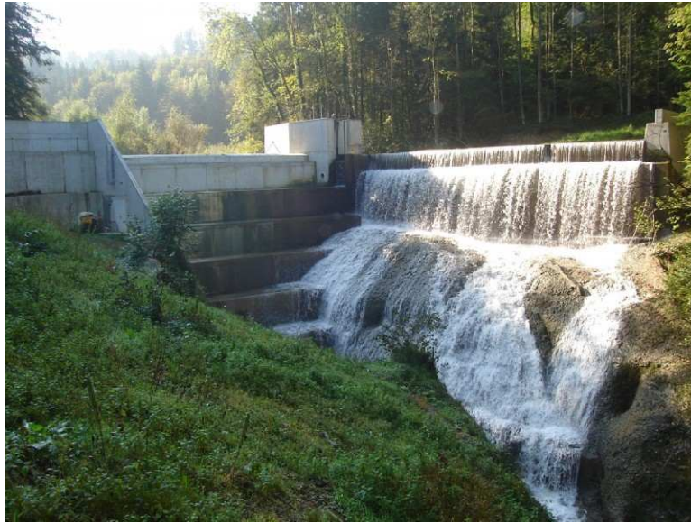
Figure 25.19: Small hydropower plant, Buchholz, Switzerland. (36)
