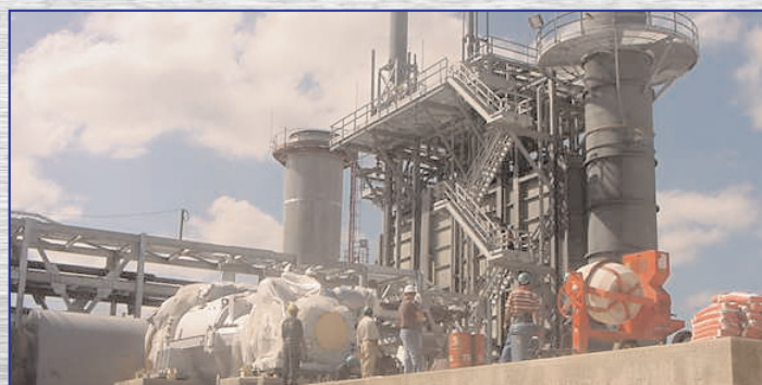
Gas Turbine (Bogue Power Plant Montego Bay)
