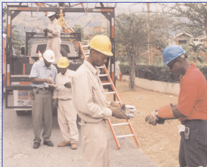
Employees assisting each other, one with preform, the other with D Iron creating a Spool Insulator for the Power Lines.
