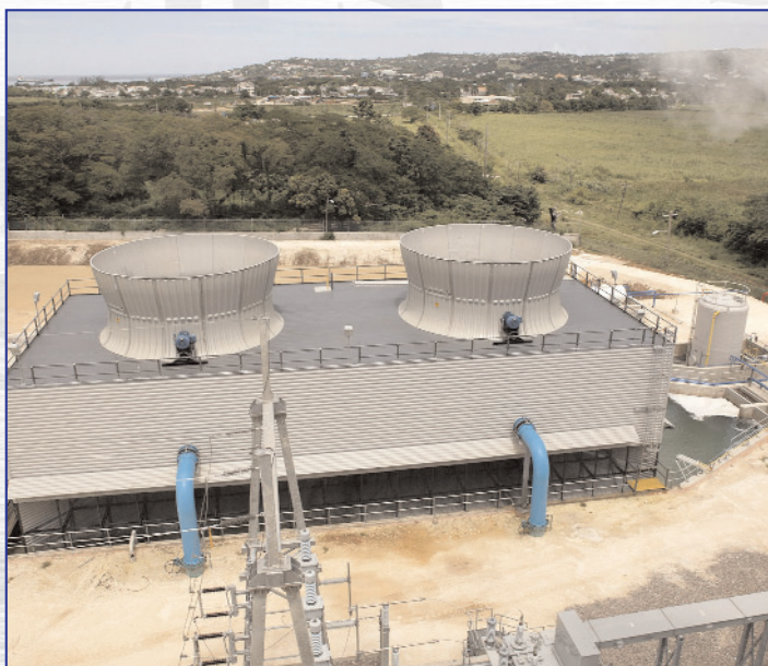
Section of Bogue Power Plant combined cycle.
