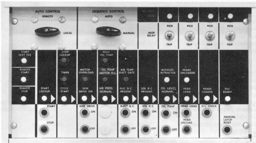
Figure 3-5. Power Sequence Control Panel
