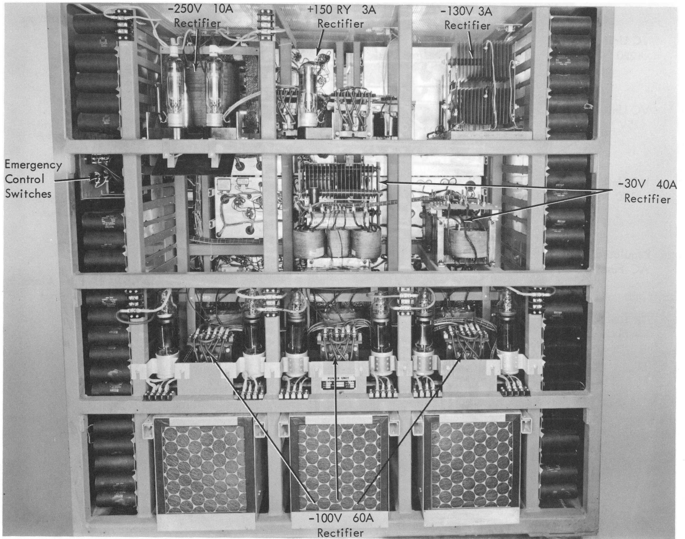
FIGURE 51-5. IBM 741 (POWER FRAME 2) (FRONT VIEW)
